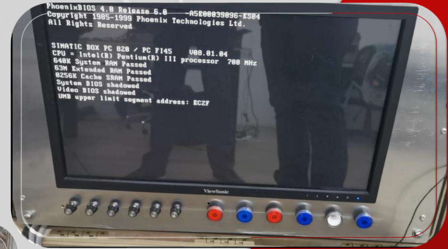
Upgrade de sistema PLC
